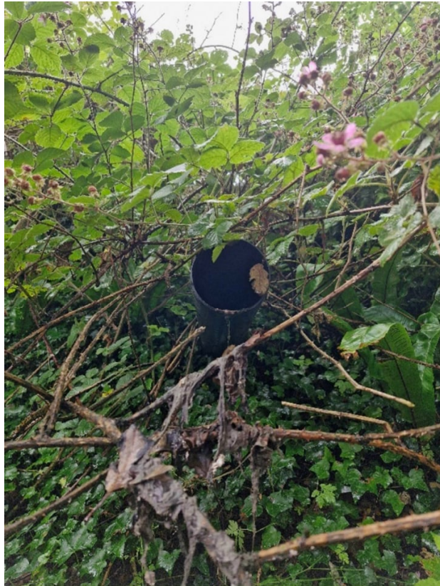
Plate 4 Pipe outflow at SW1 sampling location
